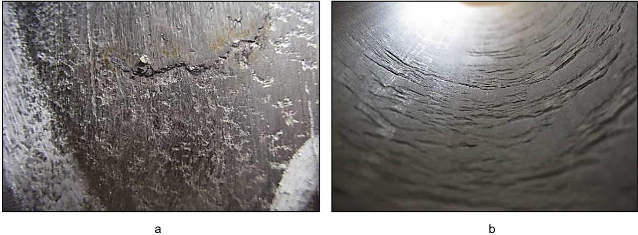
Figure 5. Appearance of defects (breaches in integrity) on the inner surface of the pipe: a – longitudinal cracks; b – rough 'ripples'.
